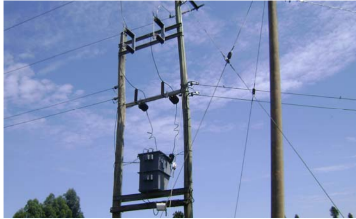
Figure 4.4: Existing 33 kV line
